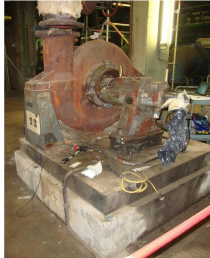
The in situ non connected pump
